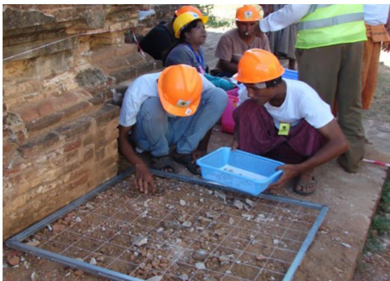
Grid for retrieving small fragments of stucco decorations at a pagoda in Bagan, Myanmar, 2016. Photo: ICCROM.
