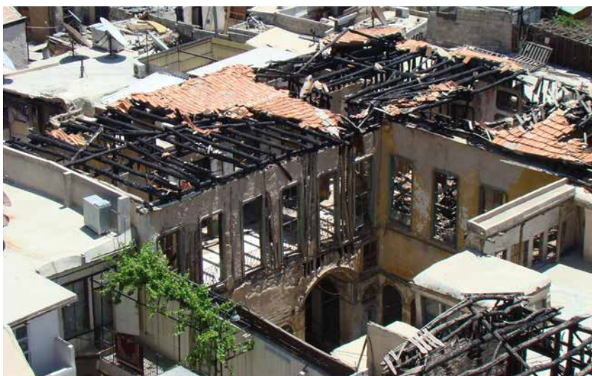
Heritage building damaged by fire (Image courtesy of Firas Otman).
