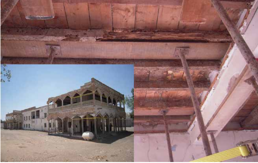
Heritage building has its wooden structure weakened by termites (Image courtesy of José Luiz Pedersoli Jr.).
